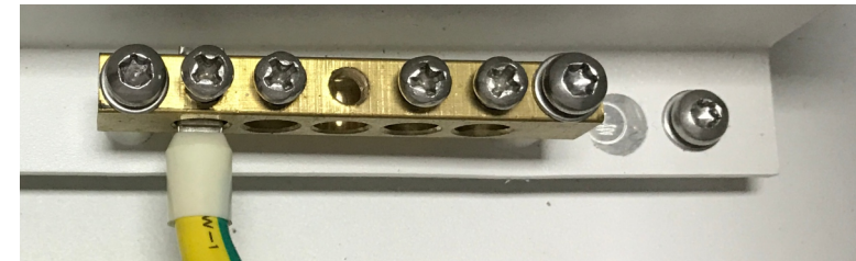
Figure 3.9 Grounding terminal block on the metal bracket
