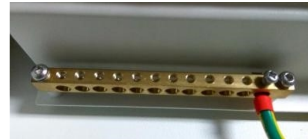
Figure 3.9 Grounding terminal block on the metal bracket
